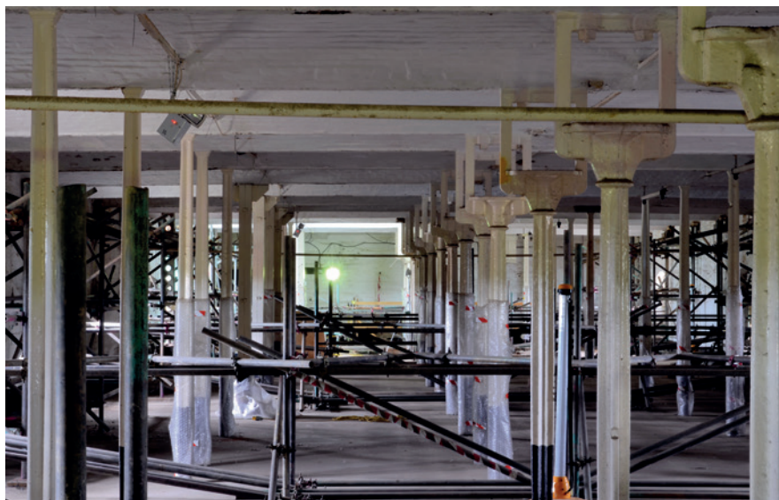
The interior of the flax mill: the line of short cast iron columns once held the drive shaft to power the looms.
