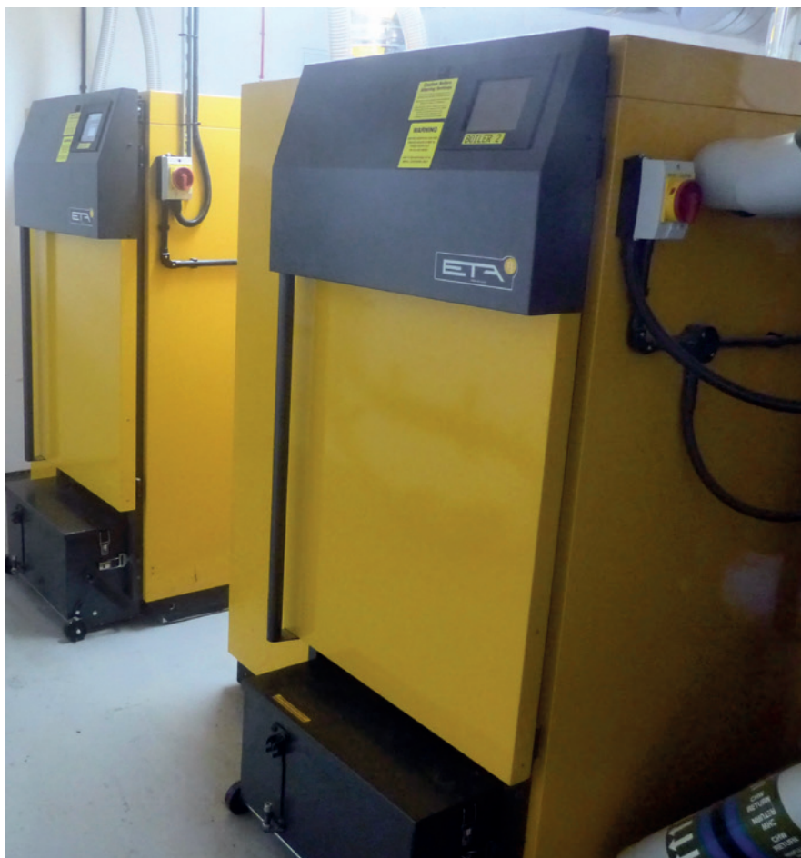
Upton House, Warwickshire was using 25,000 litres of oil each year before the installation of two wood pellet boilers, which are now saving £6,000 a year on energy bills and 55 tonnes of CO 2 emissions.
