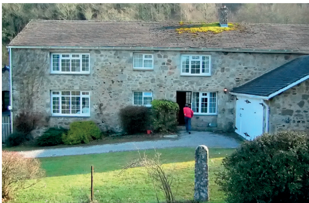
North-west facing granite wall in Drewsteignton, Devon: one of two internally insulated solid walls featured in the Building Performance Survey, this 600mm granite wall had been internally insulated with 100mm of polyisocyanurate board with an air gap and a plasterboard and gypsum skim finish.
