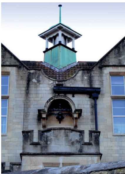
A 1930s copper cupola providing passive stack ventilation on a former school building in Bath
