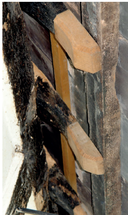
These rafters have been restored to their original overhang, greatly improving protection of the wall below.
