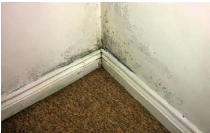
Damp and mould caused by poor external wall insulation (Photo: Centre for Sustainable Energy)
