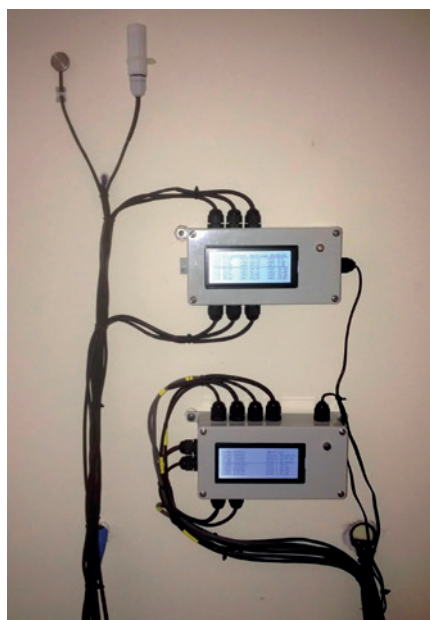
Monitoring equipment installed on the internally insulated granite wall at Drewsteigton
