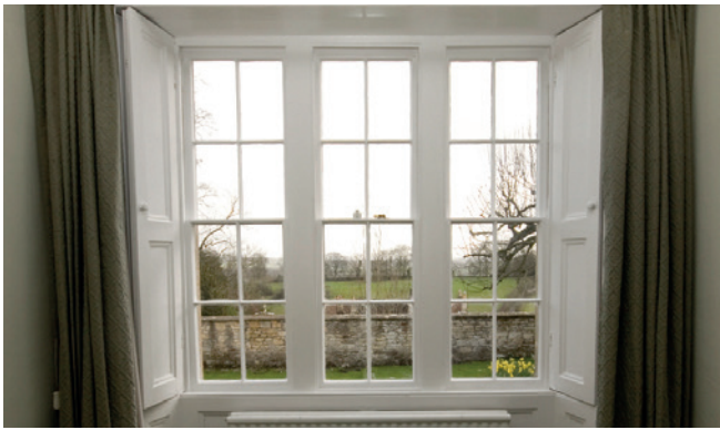
Most of the heat loss through this Georgian sash window was eliminated simply by draught-stripping. The restored shutters and heavy curtains also enabled the window to be insulated after dark.
