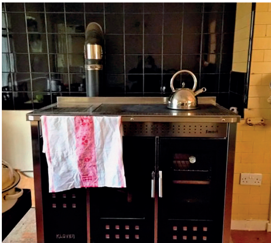
Used to heat the property and for cooking, the wood pellet range cooker trialled at Hafod y Llan in Snowdonia reduced fuel costs considerably and demonstrated that wood pellet ranges are a viable alternative to the oil-fired models used in many similar properties.
