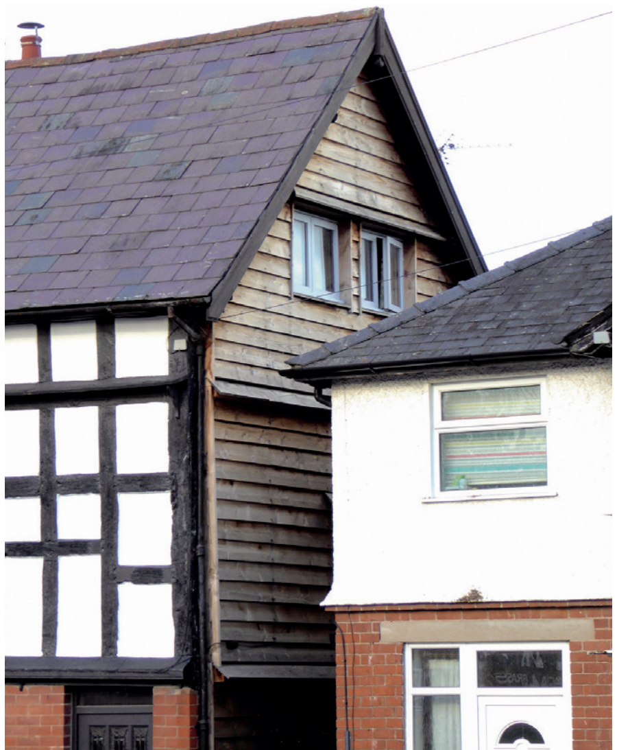
The severely degraded timber framed end wall has been strengthened and protected behind weatherboarding, with a layer of breathable multi-layer insulation included.
