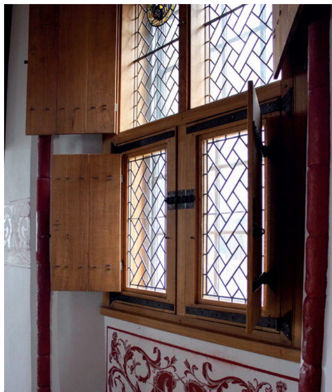
Stirling Castle, Scotland: crafted secondary glazing and shutters have been installed as part of the restoration works in the royal apartments.
