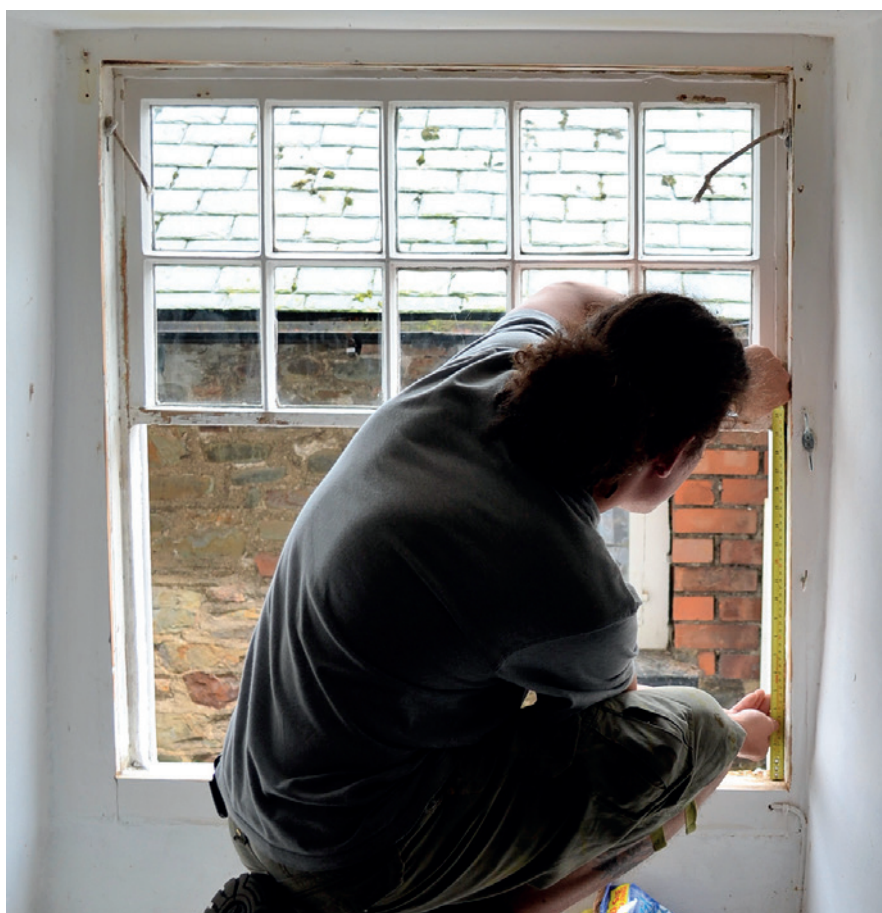
Above, draught-stripping sash windows at Clovelly, Devon as part of the programme of EPC improvement measures and, top left, simple secondary glazing fitted to a casement window. (Photos: Jonathan Taylor)
