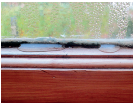
Condensation on a window pane is often a good indicator of inadequate ventilation.
