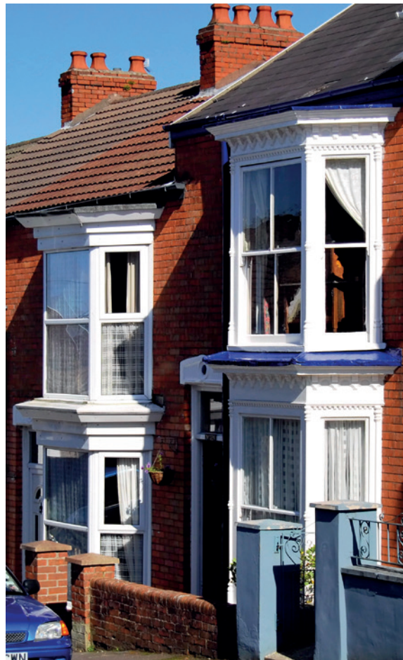
Solid brick walls, bay windows and tiled roofs in a typical Edwardian terrace. Venting top and bottom, the original vertical sliding sashes (right) offer controlled and highly efficient air circulation when retrofitted with draught seals.
