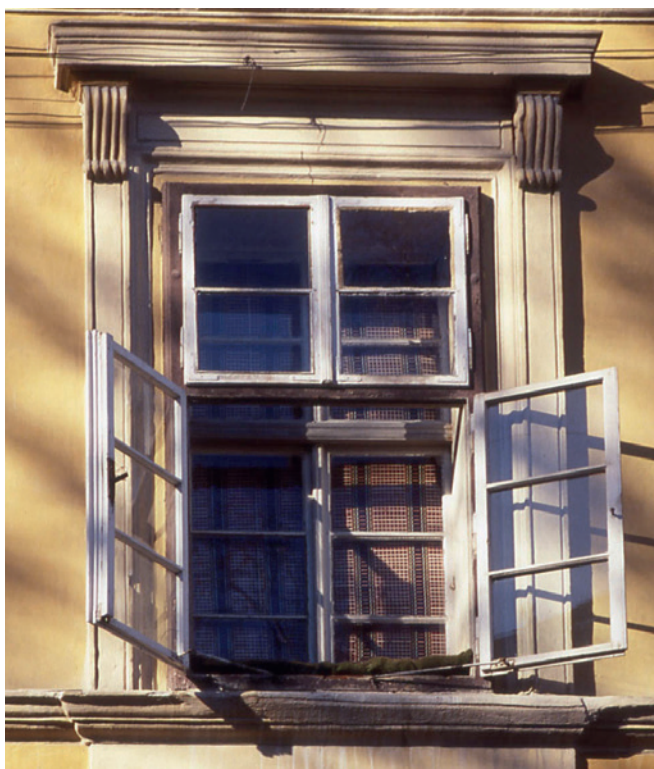
Sibiu, Romania: historic double windows, typical of those found throughout Central and Eastern Europe
