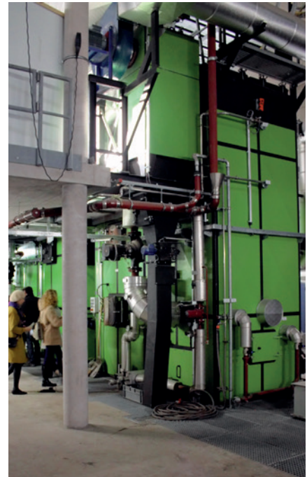
Lörrach, Baden-Württemberg, south-west Germany: biomass-fuelled urban-district heating plant. District energy systems, whether for heating/cooling or electricity, are more cost-effective and sustainable and avoid impacting on the heritage significance of individual buildings.
