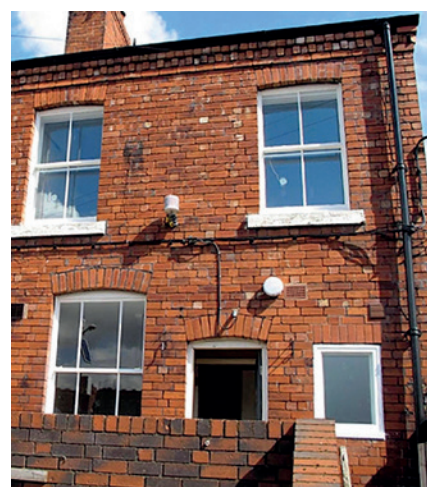
Victorian end-of-terrace in New Bolsover, Derbyshire before (above) and after (below) installation of loft insulation, secondary glazing, internal wall insulation and insulation of the suspended timber ground floor. These thermal improvement measures increased the building's SAP rating from E (46) to C (73).
