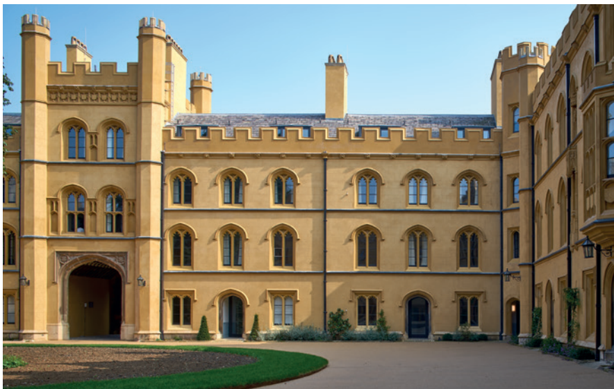
Originally the façades facing the courtyard were all rendered with Roman cement, later repairs were executed in cement, and they have now been re-rendered using a more permeable hydraulic lime painted with limewash (above).
